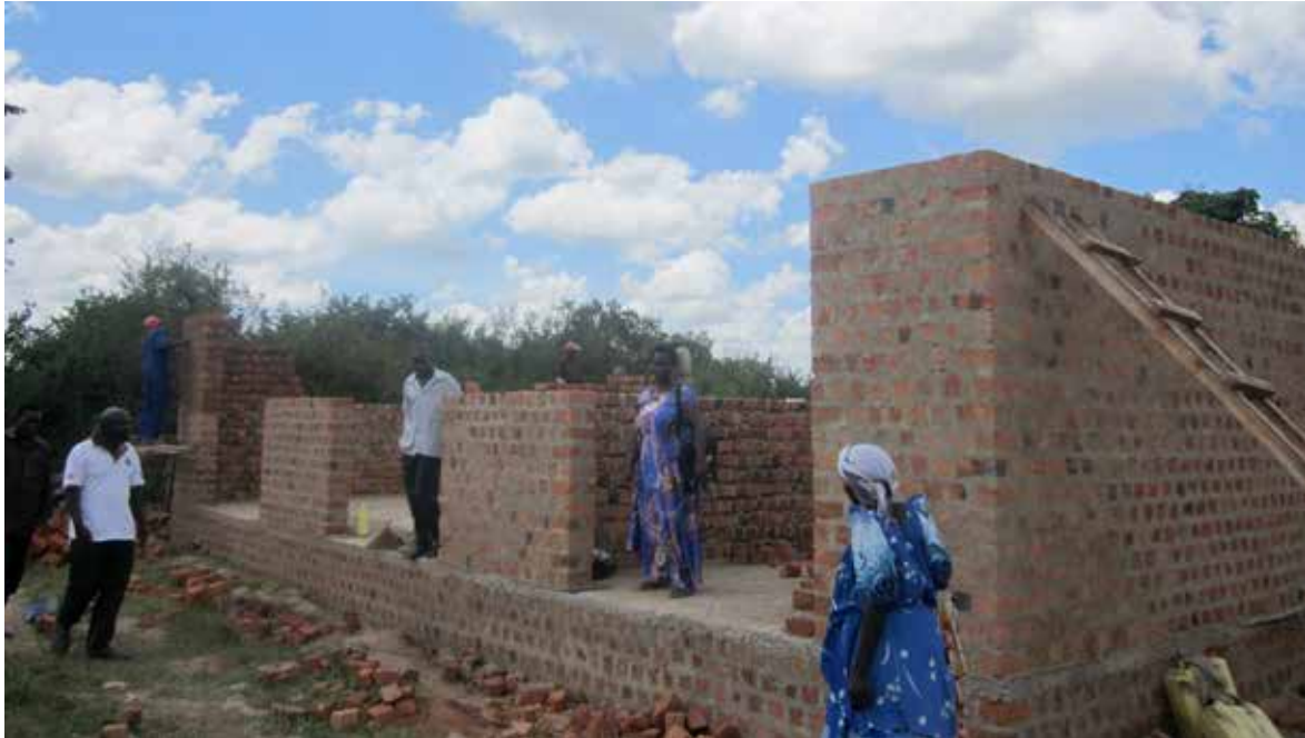
The group is building a storage facility to bulk their harvested maize.
